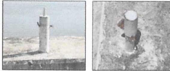
Figure 6. The crest Settlement staple cover is not installed and the padlock is broken
